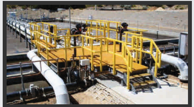
Tuas Desalination Plant, Singapore
