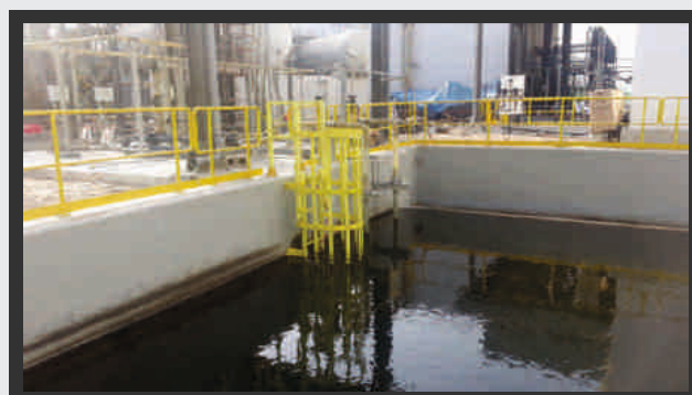
Ghubra Water Power Plant, Oman
